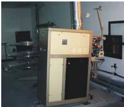
FP 50 A projector and FT 3 M platter system in a SF Cinema Bangkapi projection room
