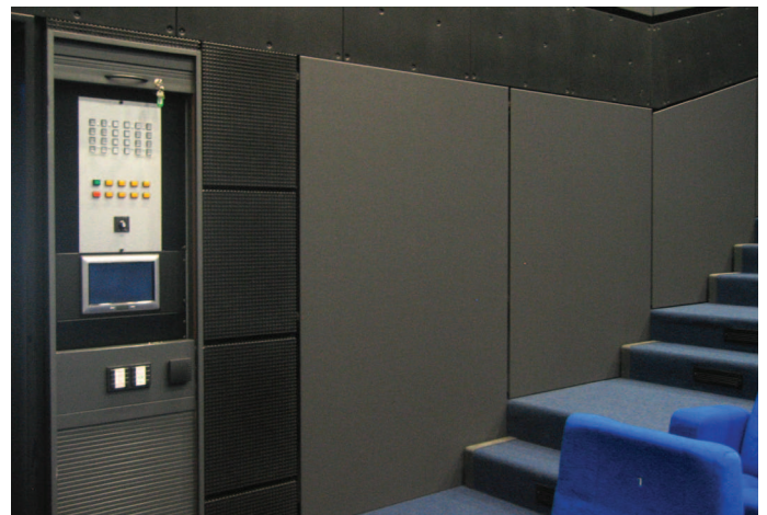
Figure 4: Control panel in the auditorium
